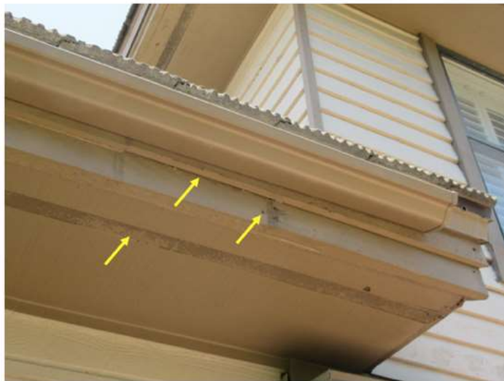
View of typical fascia dry-rot decay and partially sealed soffit vent.
